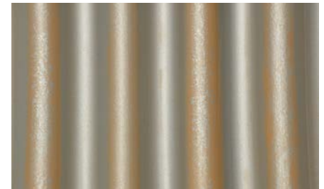
† Streaked Galvanized Rust®
